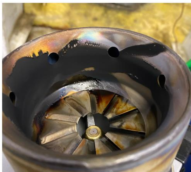
Figure 15: Carbon deposit build-up on the blast tube of an incorrectly converted burner
